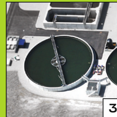
EFFLUENT TREATMENT FACILITIES
